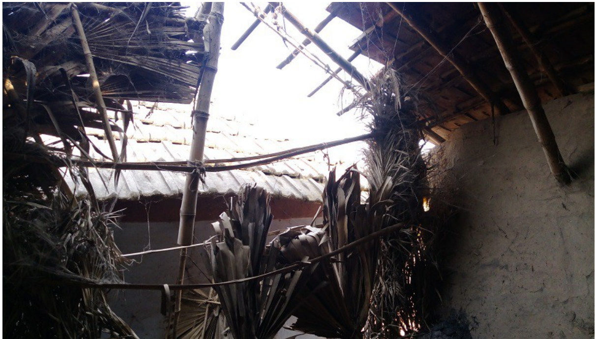
Annexure 1: The broken part of Lukhi Murmu's house
